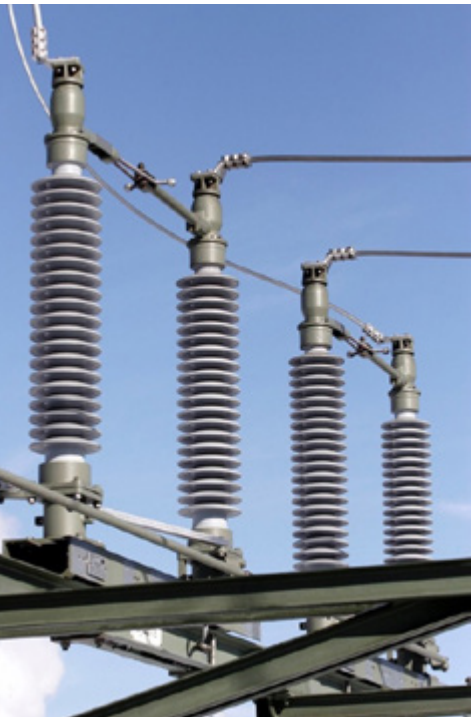
Silicone composite insulators support high-voltage equipment in an outdoor substation, where hydrophobic, weather-resistant housings contribute to long-term insulation performance. (Source: WACKER)
