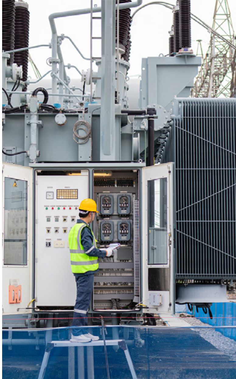
The cheapest transformer is the one you don't have to buy. Digital monitoring and grid-enhancing technologies stretch the capacity of assets already in the ground. Credit: [JD Studio / Adobe Stock]
