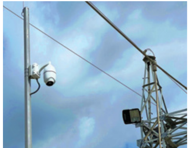
Figure 1. Pan-Tilt-Zoom Cameras used to monitor operations and asset conditions.
