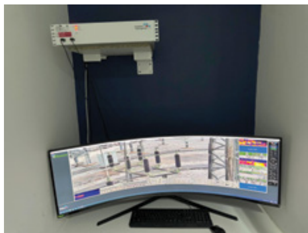
Figure 3. Substation hardened servers used for local video and data analysis and storage.
