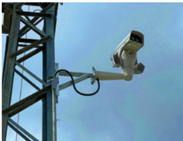
Figure 2. Thermal-visual sensors on Pan-Tilt units for automated asset monitoring and detection of hot spots.
