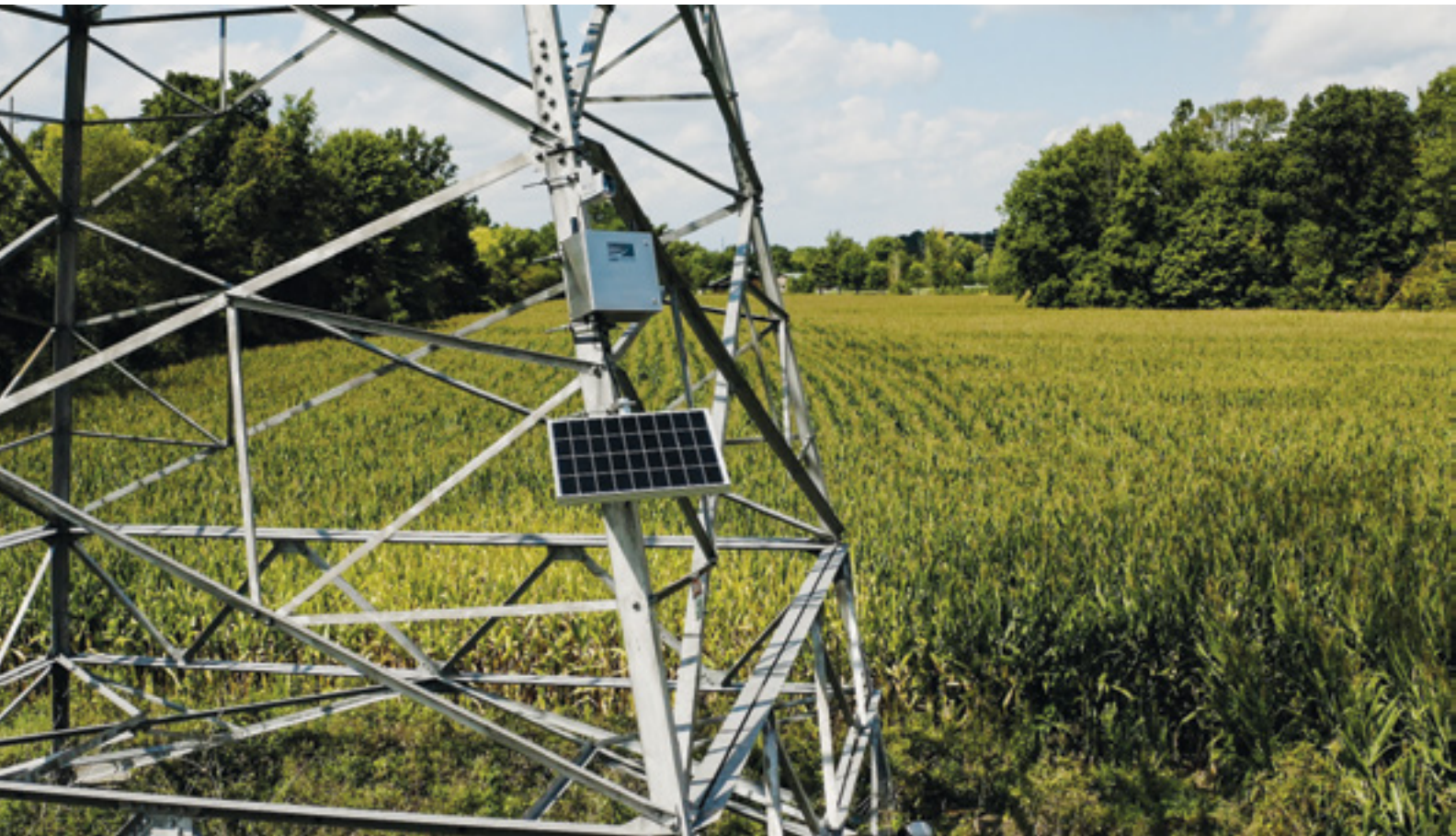
A LineVision non-contact sensor is installed on an AES transmission tower. Source: LineVision.
