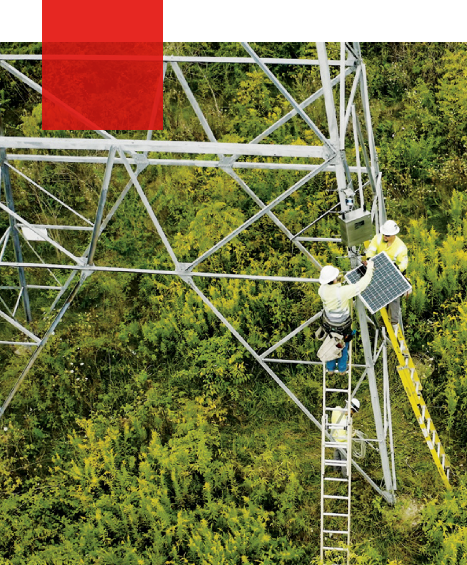
AES lineworkers install a LineVision non-contact sensor on a transmission tower. Source: LineVision.
