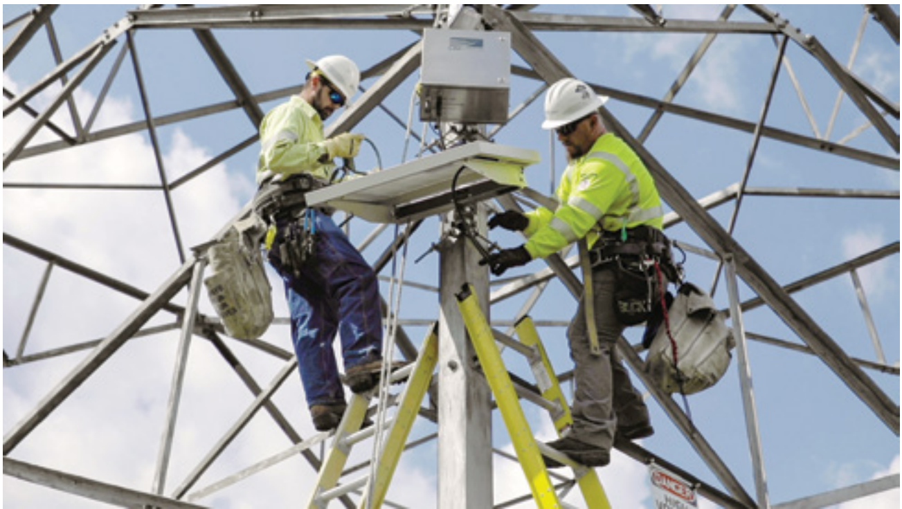
Lineworkers secure a LineVision non-contact sensor on an AES transmission tower. Source: LineVision.
