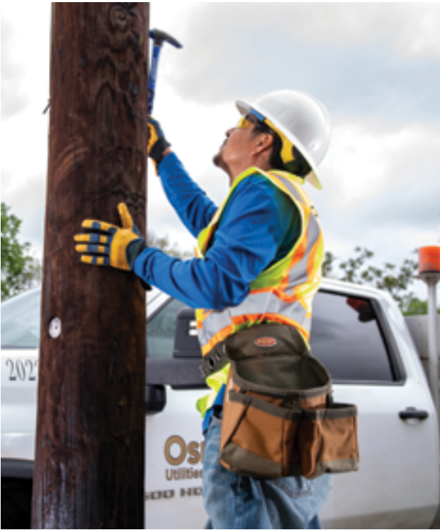
Performing a sounding inspection on a wood utility pole. Credit: Osmose Utilities Services
