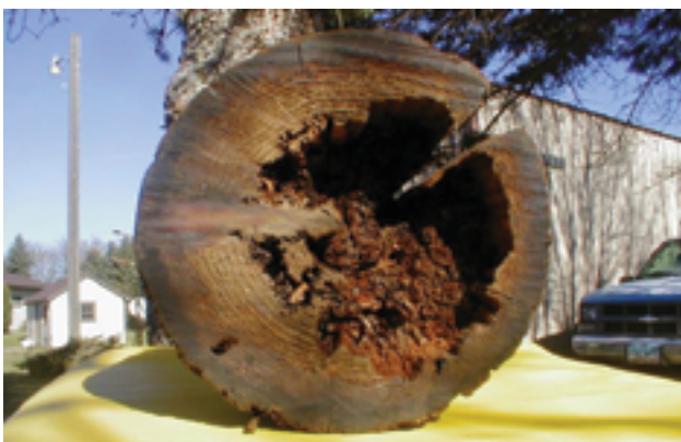
Shows the decay pattern of a thin sapwood pole because these poles decay from the inside-out Credit: Osmose Utilities Services
