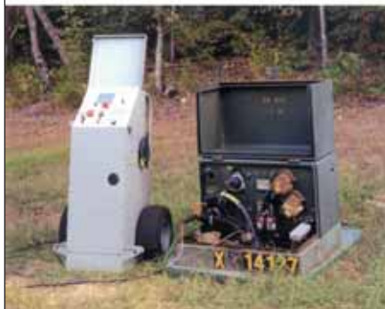
Portable Fault Locating
