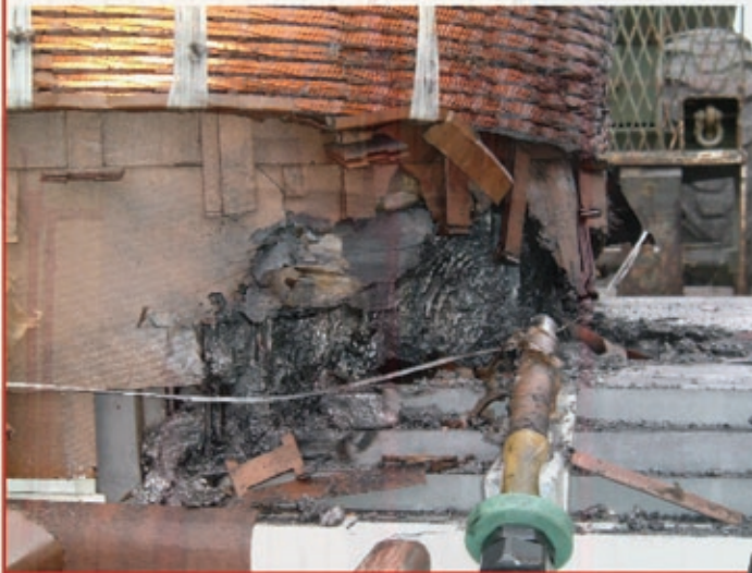
Core damage at bottom of center limb (cluster1)
